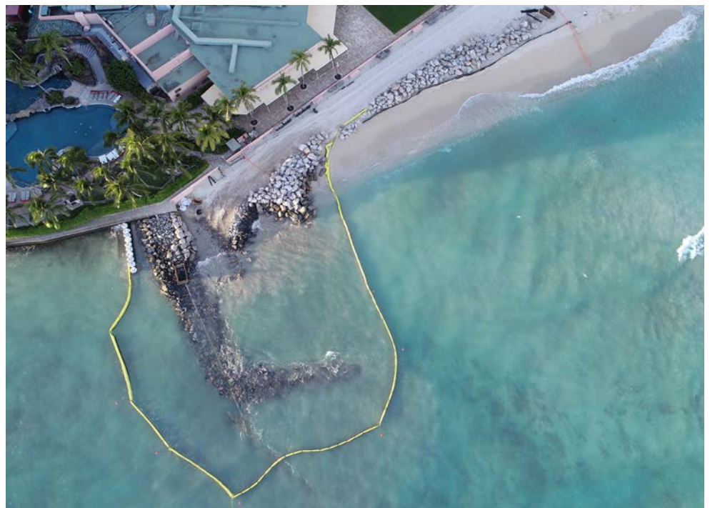
Royal Hawaiian groin under construction (May 29, 2020). Note the outline of "L" shape of the groin on the seaward end.
