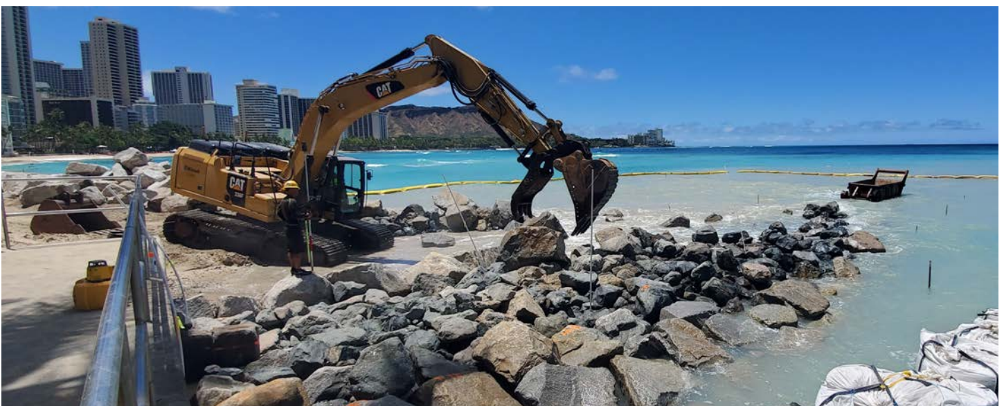
Royal Hawaiian groin under construction (June 1, 2020). Rocks are being placed at the landward stem of the groin.
